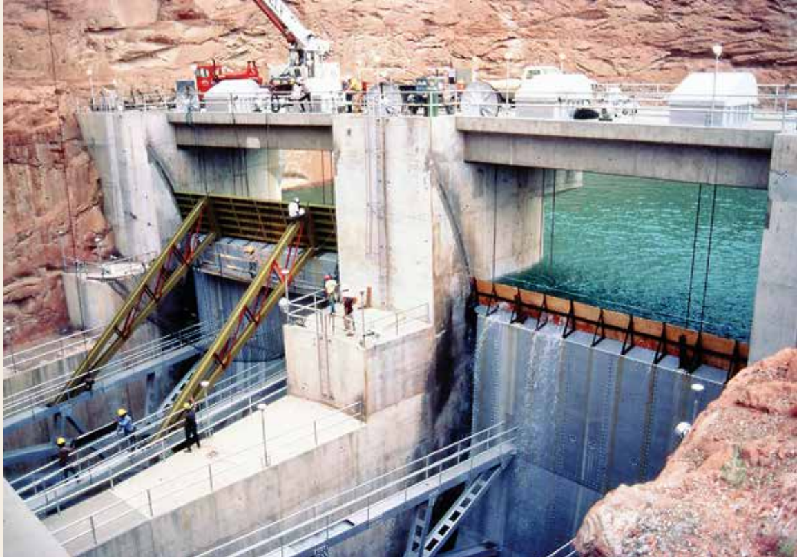
Crews work to raise the top of the spillways on Glen Canyon Dam. Plywood flash boards are visible on the right gate. Photo: Bureau of Reclamation
