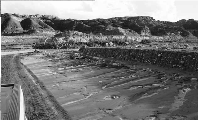
Levee damage from the October flood. Photo courtesy Greg Squires—NPS
