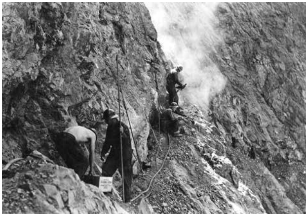
Construction of River Trail by CCC enrollees. Enrollees working on ledge. Blasting area. Circa 1935. NPS.
